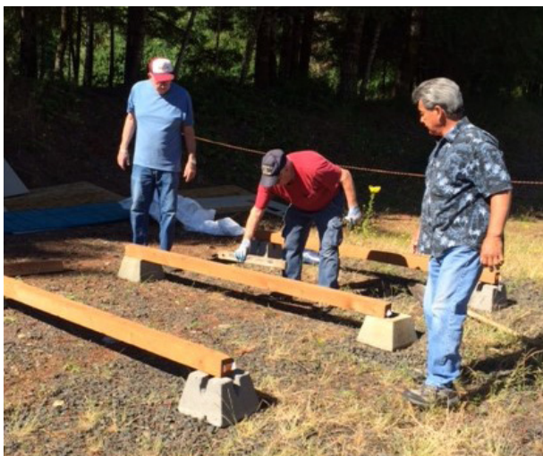
Clay Long, Dave Brown and Terry Knobloch laying the foundation of the garden Shed.
